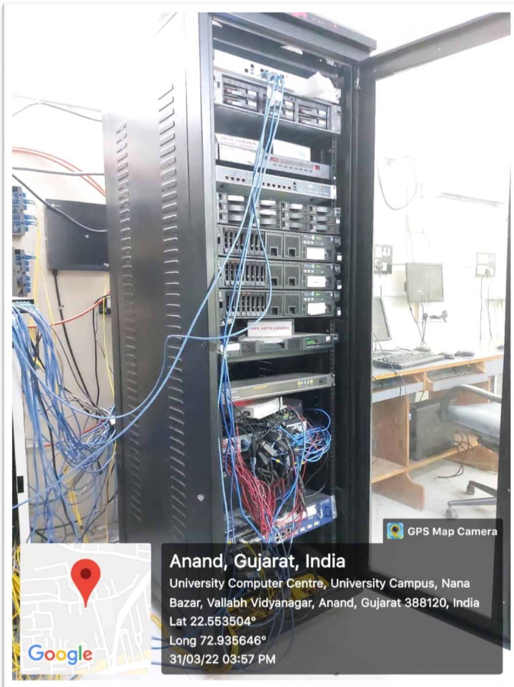
University Computer Centre – Servers
