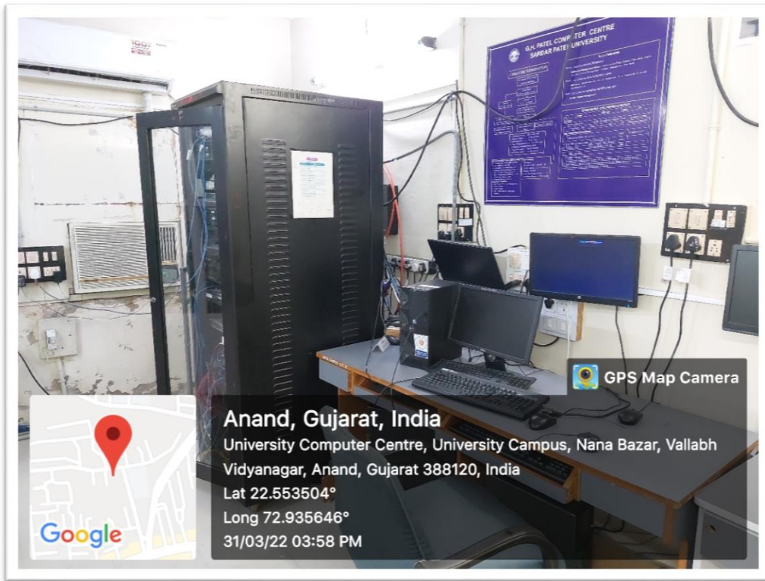
University Computer Centre – Server Room
